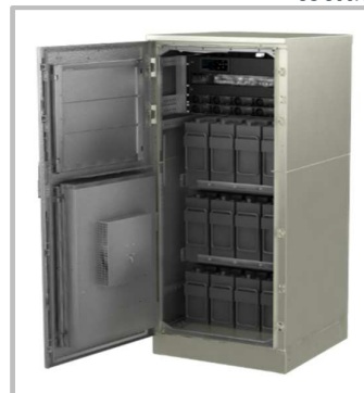
FLATPACK2 SYSTEM IN TYPE 3 OUTDOOR CABINET
